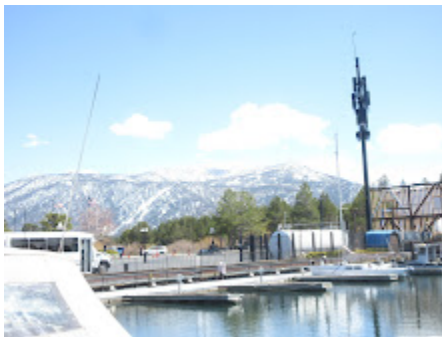
Wireless Facilities Tower at Tahoe Keys Marina, facing Southeast, 4-16-20.JPG 4942K
